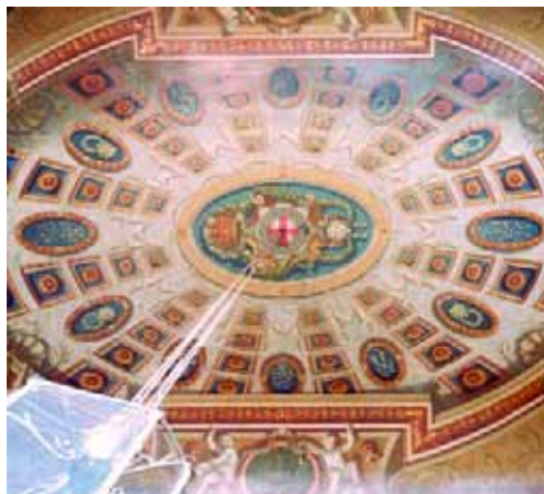
Fig. 18. General view of the ceiling of the Queen's Staircase, Hampton Court Palace. The image was made as part of a rectified photography survey and has a pair of superimposed fine cross-hairs which are not part of the painted image. © Crown copyright: Historic Royal Palaces
